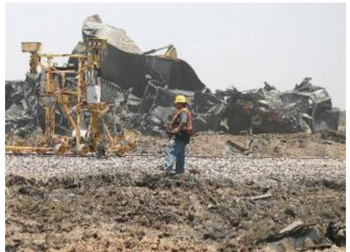
Union Pacific crews work to repair damaged track at the site of a head-on train collision on Monday, June 25, 2012, near Goodwell, Okla. Two Union Pacific locomotives collided on June 24, 2012, killing two crew members and a conductor. (AP Photo/The Guymon Daily Herald, Shawn Yorks)
