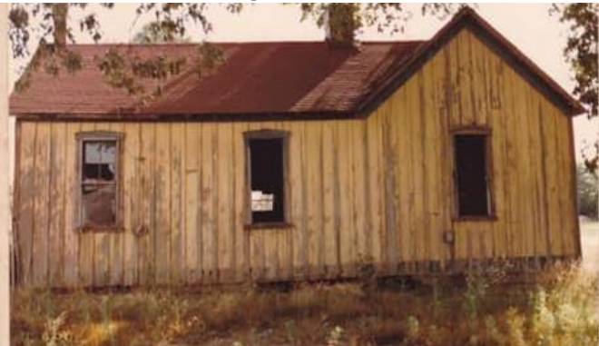
Left side view showing a non-standard "L" addition
