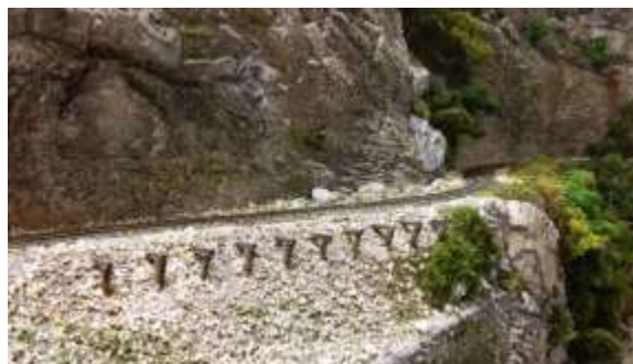
Trestle bents poke through the backfill at the retaining wall in the Doe River Gorge, a historical detail included in the modeled portion of the gorge
