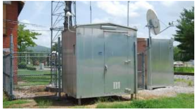
CXS still maintains signal equipment on site
