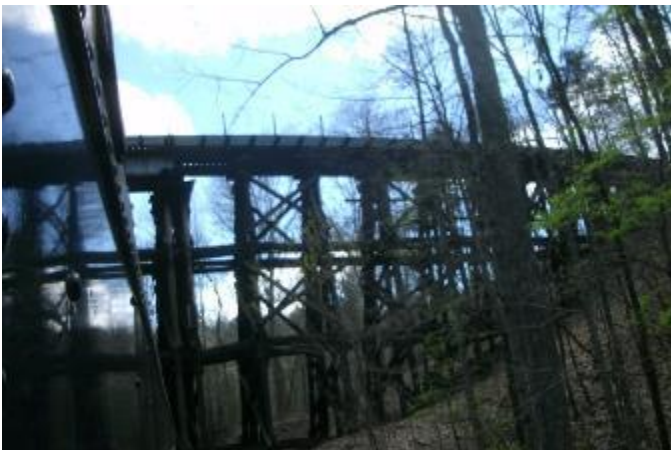
The trestle carries the line over itself after completing 1 3/4 loops upon itself.
