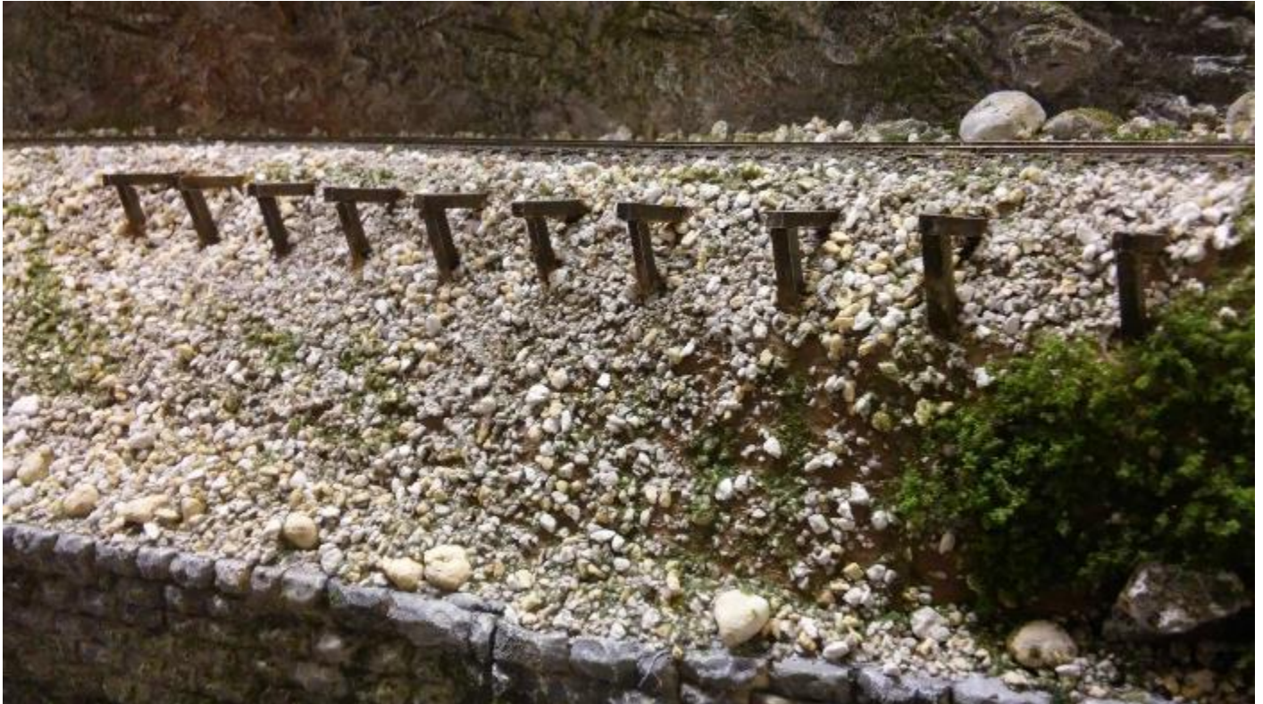
TRESTLE BENTS PEAK OUT FROM UNDER THE FILL IN THE DOE RIVER GORGE
