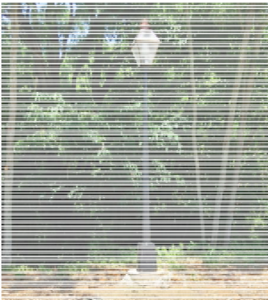
Decorative street lighting will highlight the site of the rehabilitated station. A string of street lamps like the one depicted above have already been installed.
