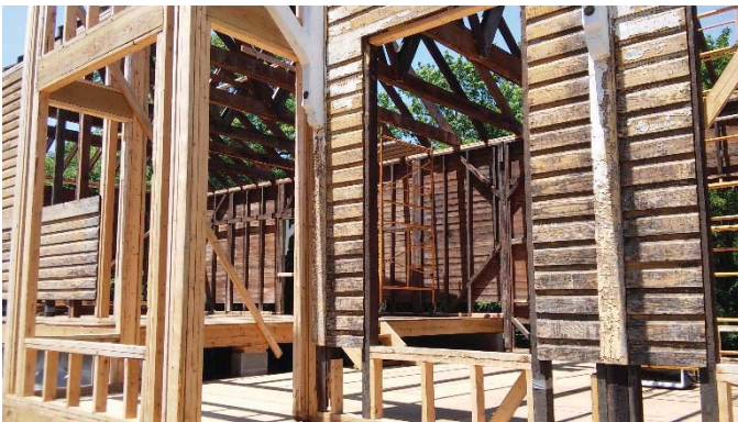
As the station is rebuilt railroad modelers have an excellent opportunity to study how the building was built. In its partially assembled state framing for the walls and flooring are easily observed.
