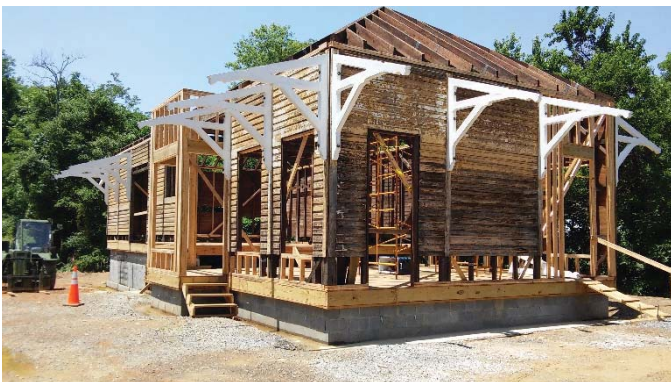
The roof trusses and rafters forming the hip roof as evident in the photos as are the eave braces.
