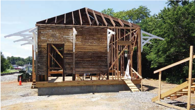
Work continues on rebuilding the former Southern RY depot that sat in Chuckey TN. The station is a Queen Anne style structure with a bay operator's window, large freight/baggage room and a segregated "Jim Crow" waiting room.
