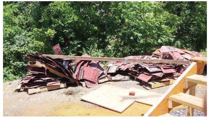
Not all the original parts of the structure are reusable. The tin ceiling tiles have been saved but appear to be in sad condition.
