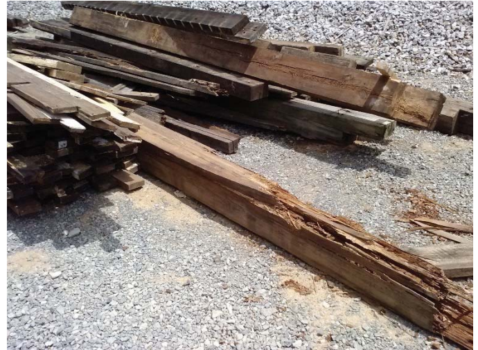
A pile of support timbers slightly worse for the wear... these have been replaced with new lumber.
