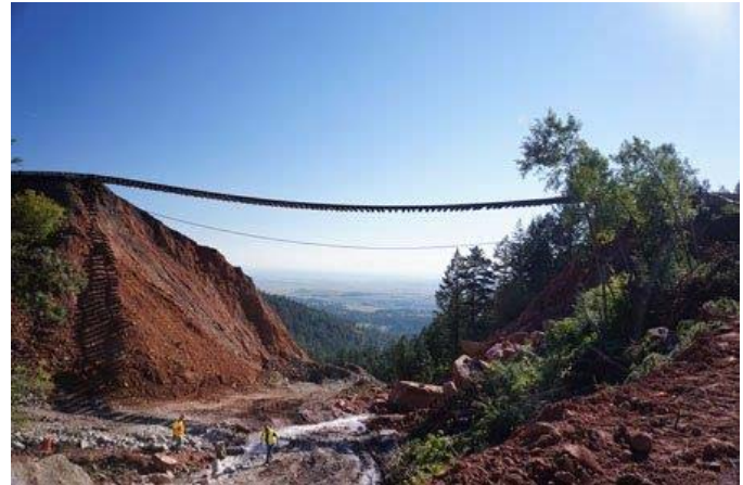
Colorado Flooding 2013 A section of track is left hanging in mid-air.
