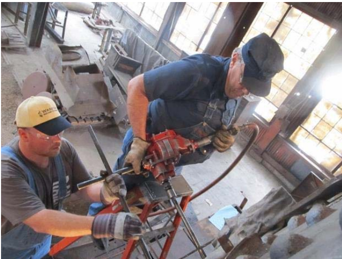
Cody Vosler of Wasatch continues welding flexible staybolt sleeves on the fireman's side of the boiler.
