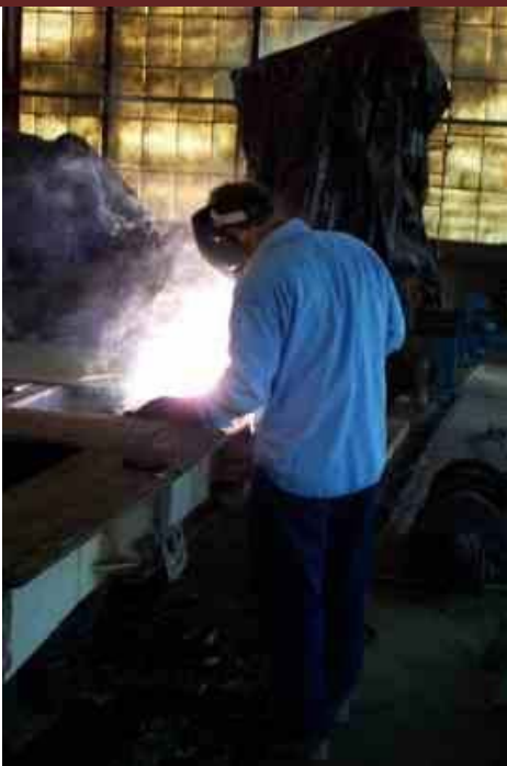
Welder-machinist Paul Anderson prepares the frame of #1003 for its new body on August 26, 2003
