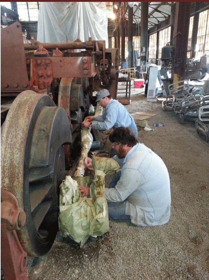
April 14, 2013. The fireman's side of the boiler with most of the flexible staybolt sleeves in place and all of the rigid staybolt holes threaded.
