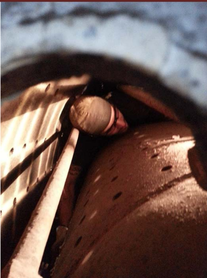
Brandon Hughett and Bill Johnson tapping staybolt holes while Kelly Barnett waits inside the firebox to catch the tap.
