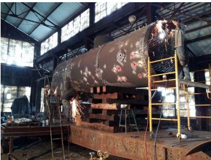
All of the firebox sheets have been fit up and welded - August 9, 2012
