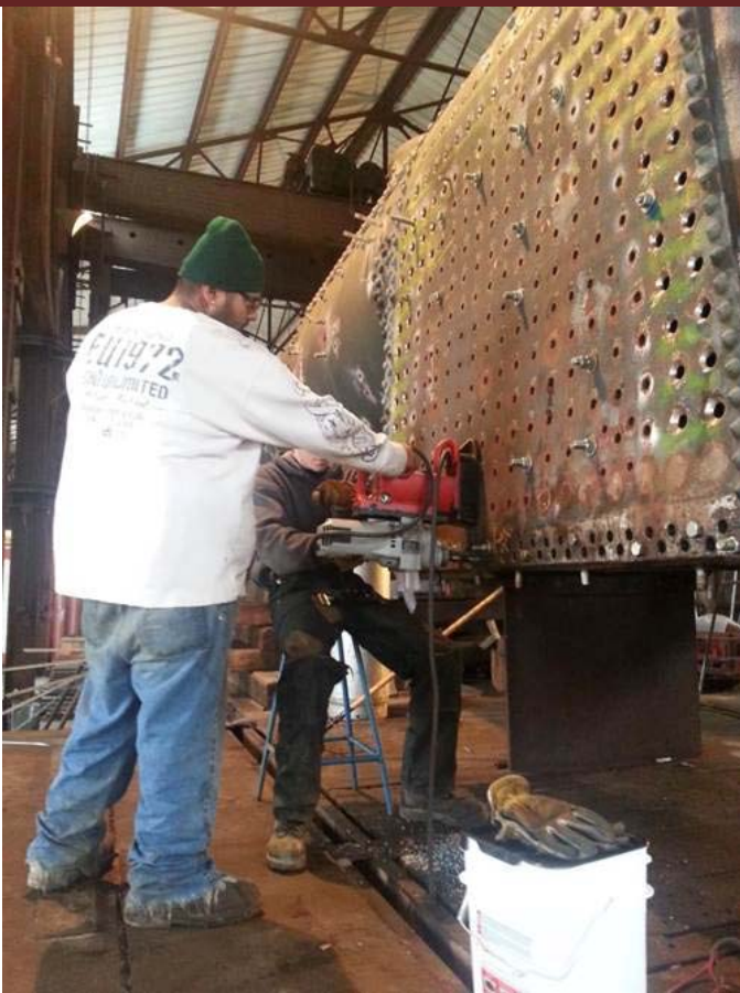
View from overhead bridge crane in the K&T Steam Shop of the smoke box being mounted on the front of K&T #14's boiler - January 29, 2013
