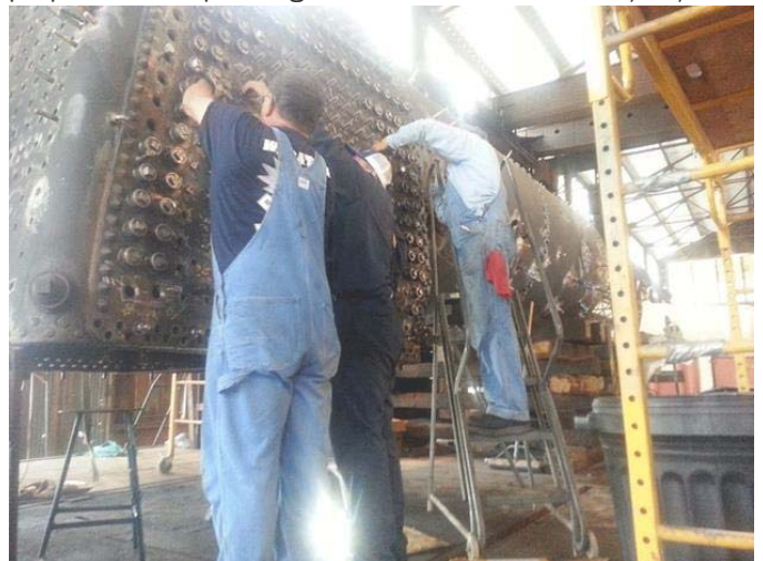
150 flexible staybolts and 300 rigid staybolts were installed June 5-9. Work was performed by Matt Cole, Brady Sanger, Kelly Barnett, Thomas Bookout and Bill Johnson.
