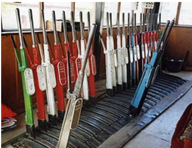
A mechanical lever frame inside the signal box at Knockcroghery in Ireland
