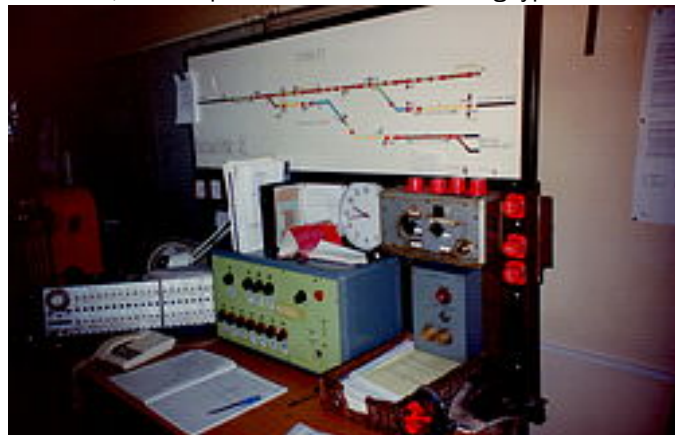
Trimley Junction IFS panel in the 1988 replacement signal box; built by BREL York
