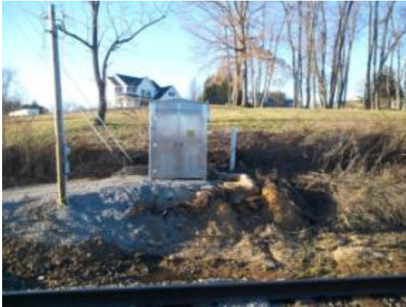
Older Installation of Relay Box
