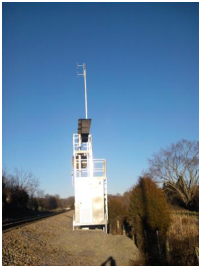
New Signal Mast with Control Box Integrated
