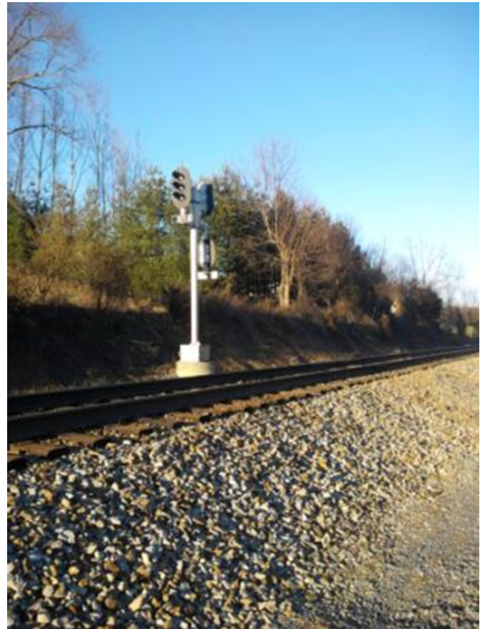
Signal Mast to be Replaced
