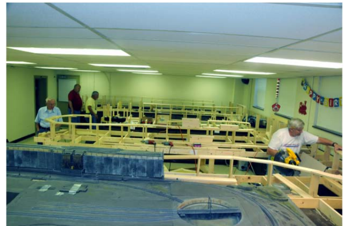
The new 1300-foot addition to the museum is rapidly being put to good use by volunteers, who are building a version of the narrow gauge East Tennessee & Western North Carolina (known affectionately as the Tweesie) from Johnson City to Cranberry, N.C.s ore banks. Four replicas of the railroad's engines as well as the special Hon3 track have been purchased; member Dwayne Swank is seen custom-fitting the support system for the track.
