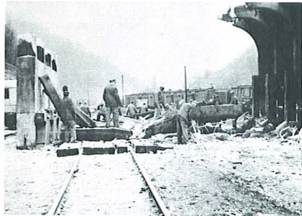
Structure down. B&B gang No. 5 beginning the task of final demolition and clean-up.
