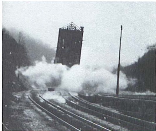
A split second after the firing. The structure has already begun to topple.
