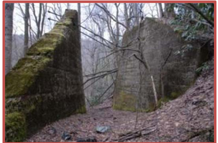
Photo 2: The State Line Hill trestle south end poured concrete abutments of the ET&WNC.
