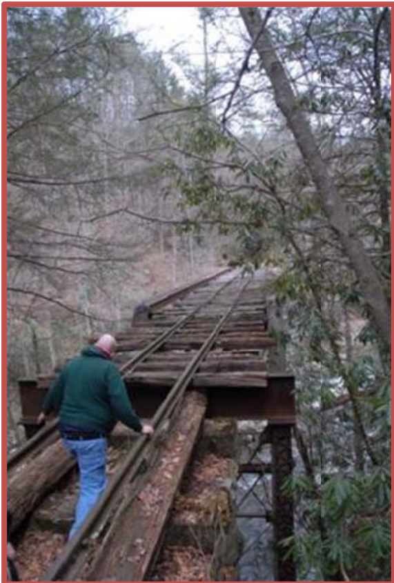
Photo 13: Gary Emmert checking the crossing situation on Steel Deck Truss bridge just north of Tunnel #4
