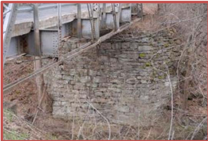
Photo 5: The well constructed stone abutment of the Blevins Steel Truss thru bridge.
