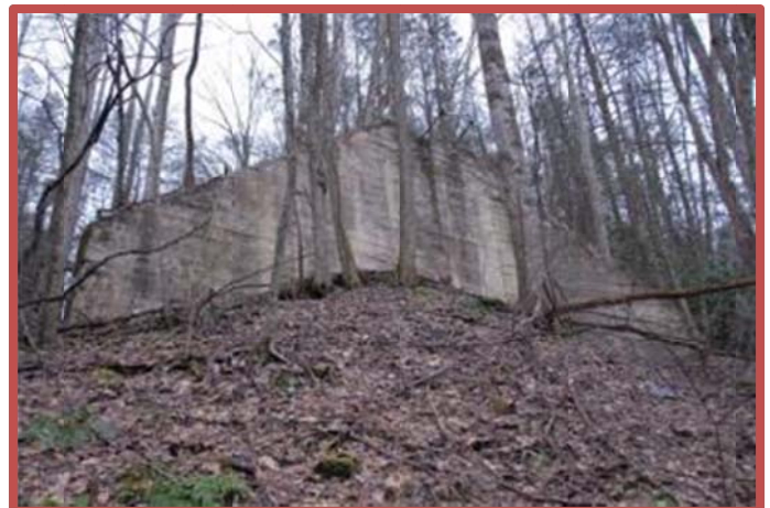
Photo 3: Looking up at the front face of the ET&WNC south side State Line Hill trestle abutment
