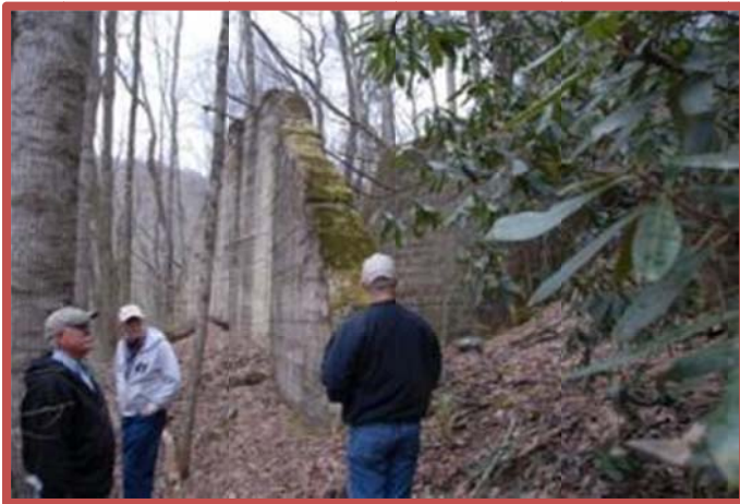
Photo 1: L to R. Jerry Turbyfill, Rich Gallaher, & Phil Sloan inspecting the south abutments of the ET&WNS State Line Hill trestle.
