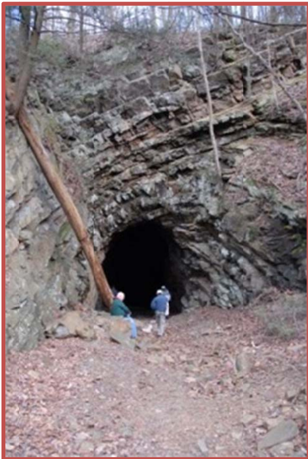
Photo 17: L to R. Gary Emmert, Phil Sloan, and Rich Gallaher at the north entrance to Tunnel #1
