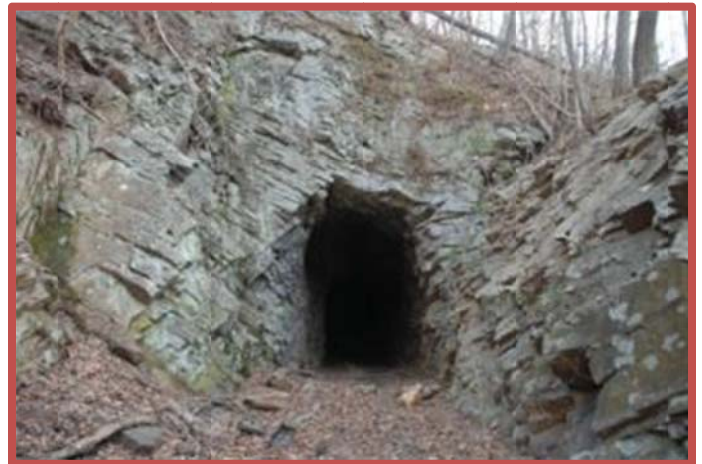
Photo 19: The south entrance to Tunnel #1. The tunnel was excavated large enough to handle standard gauge rolling stock.
