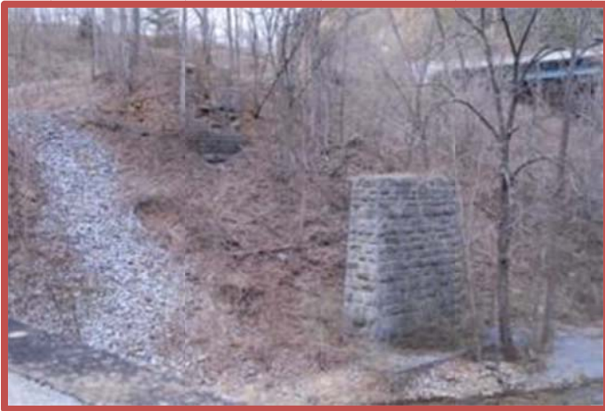
Photo 16: The stone north abutments for the ET&WNC 3-span covered wooden deck bridge viewed from the old highway bridge.
