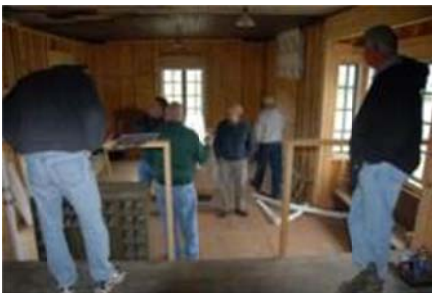
Interior of ET&WNC RR Linville Depot as it is being restored. L to R.: John Carter, Joel Shipley, Gary Emmert, Gary Rabetoy, Richard Gallaher, Jerry Turbyfill. Newland, NC
