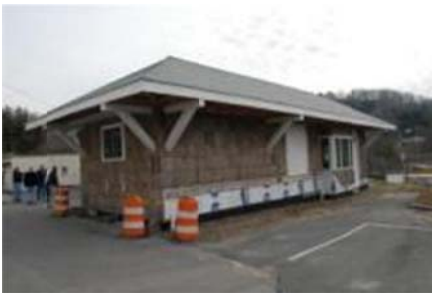
Restoration of the ET&WNC RR Linville Depot on its new site at the Avery County Museum in Newland, NC
